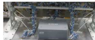
Solar Cells Control Unit (SCCU)
